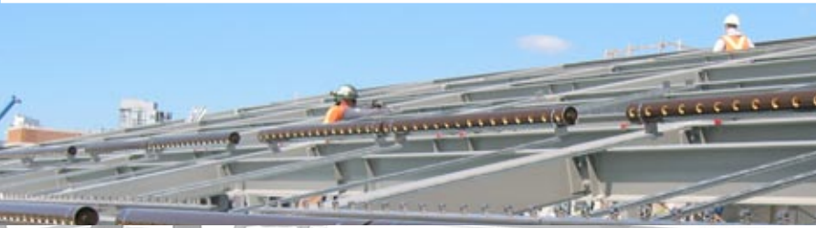
Photos of the solar array structure being installed on the roof of the Net Zero building on parcel 9.
