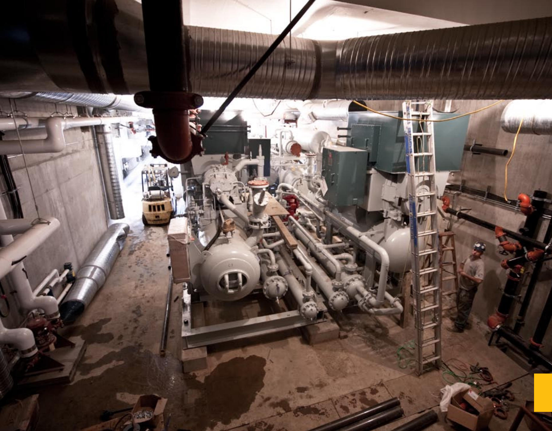
FRONT COVER The False Creek Community Energy Centre building, located under the south end of the Cambie Street Bridge, is designed as an interpretive facility to showcase the innovative use of sustainable technology. BACK COVER The inner workings of the False Creek Community Energy Centre rely largely on a giant electric heat pump that works to recover heat energy from sewage and send it back through the district heating system.
