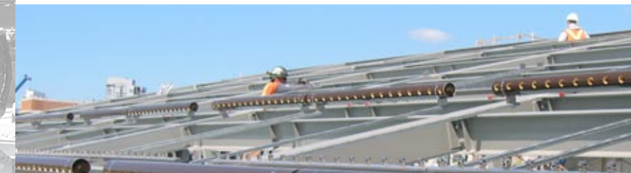
Photos of the solar array structure being installed on the roof of the Net Zero building on parcel 9.
