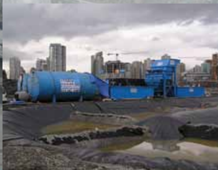
During excavation, all rainwater that fell on the site had to be captured and treated for contamination – more than 88 million gallons in total.
