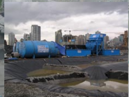
During excavation, all rainwater that fell on the site had to be captured and treated for contamination – more than 88 million gallons in total.
